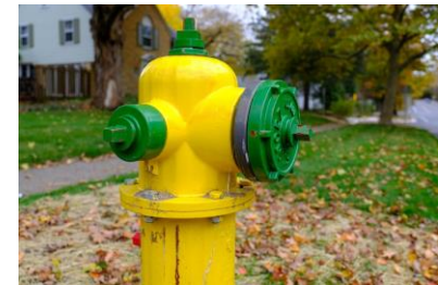
A Fire hydrant
