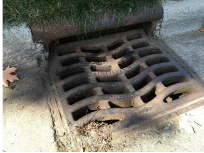
A Storm Drain
